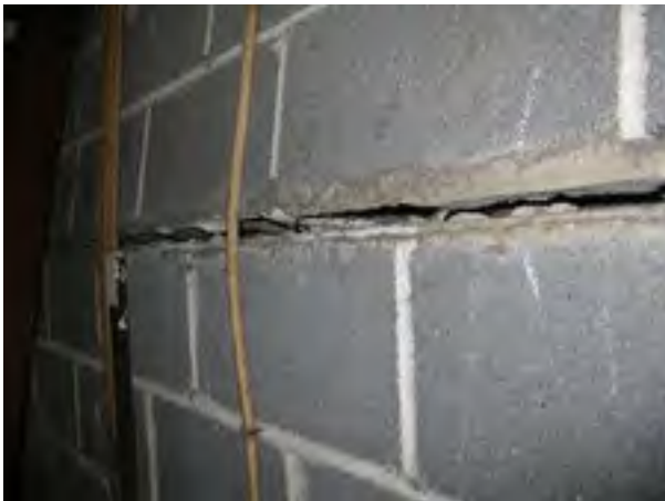
Horizontal crack at mid-height of block foundation
